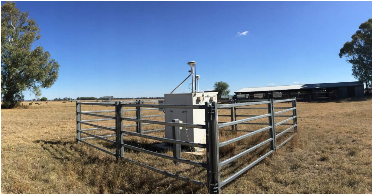
Figure 1: TEOM installed at Flixton property
